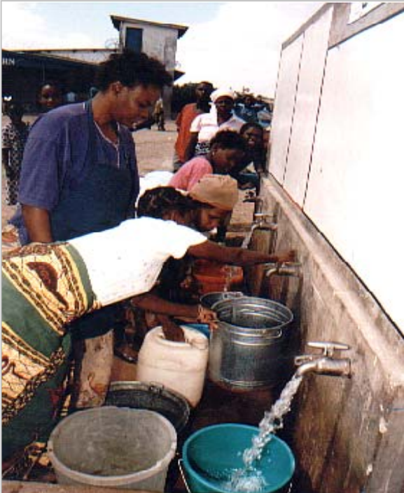
Installed communal water points
